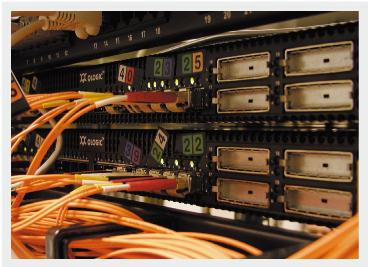
SAN network infrastructure
