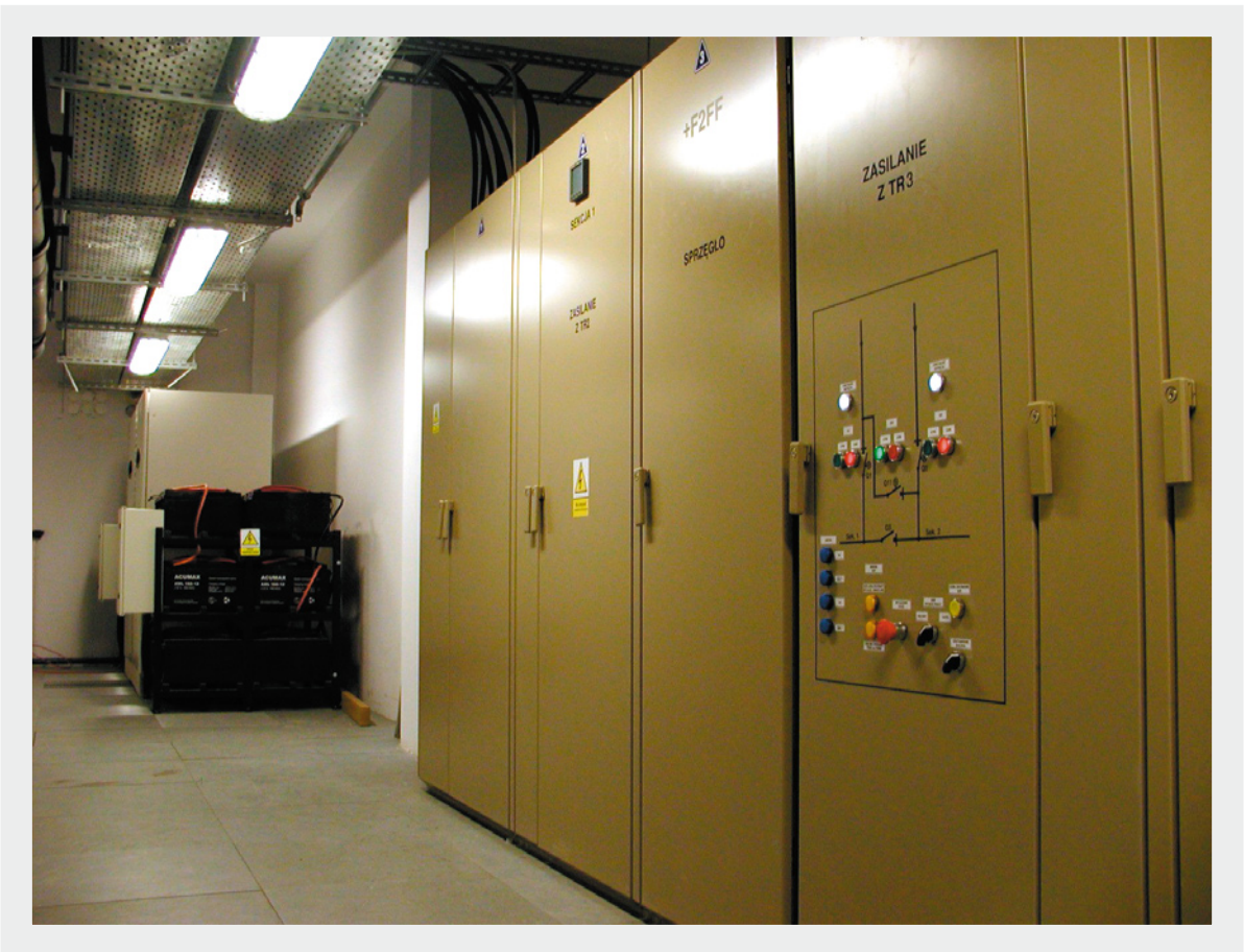
Power switching station and UPS system
