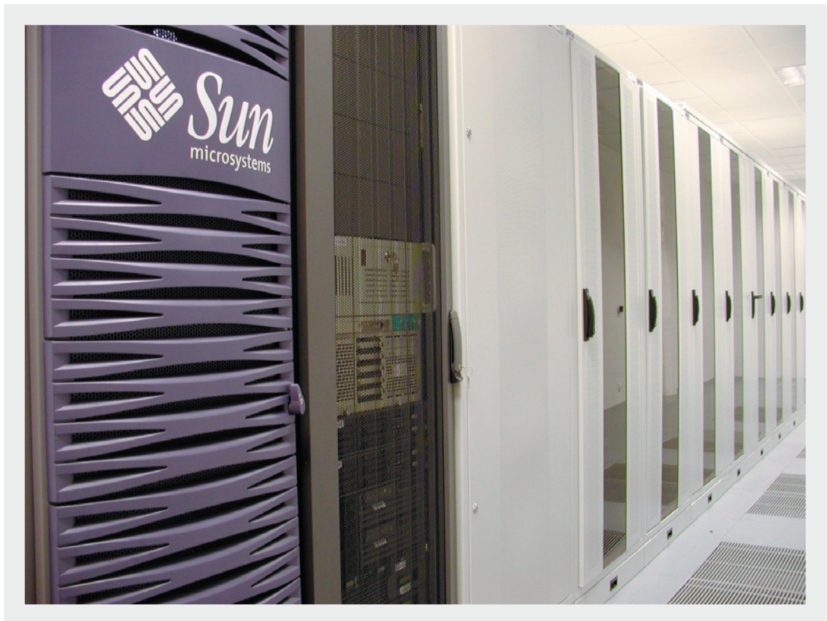
The Comarch Data Center
