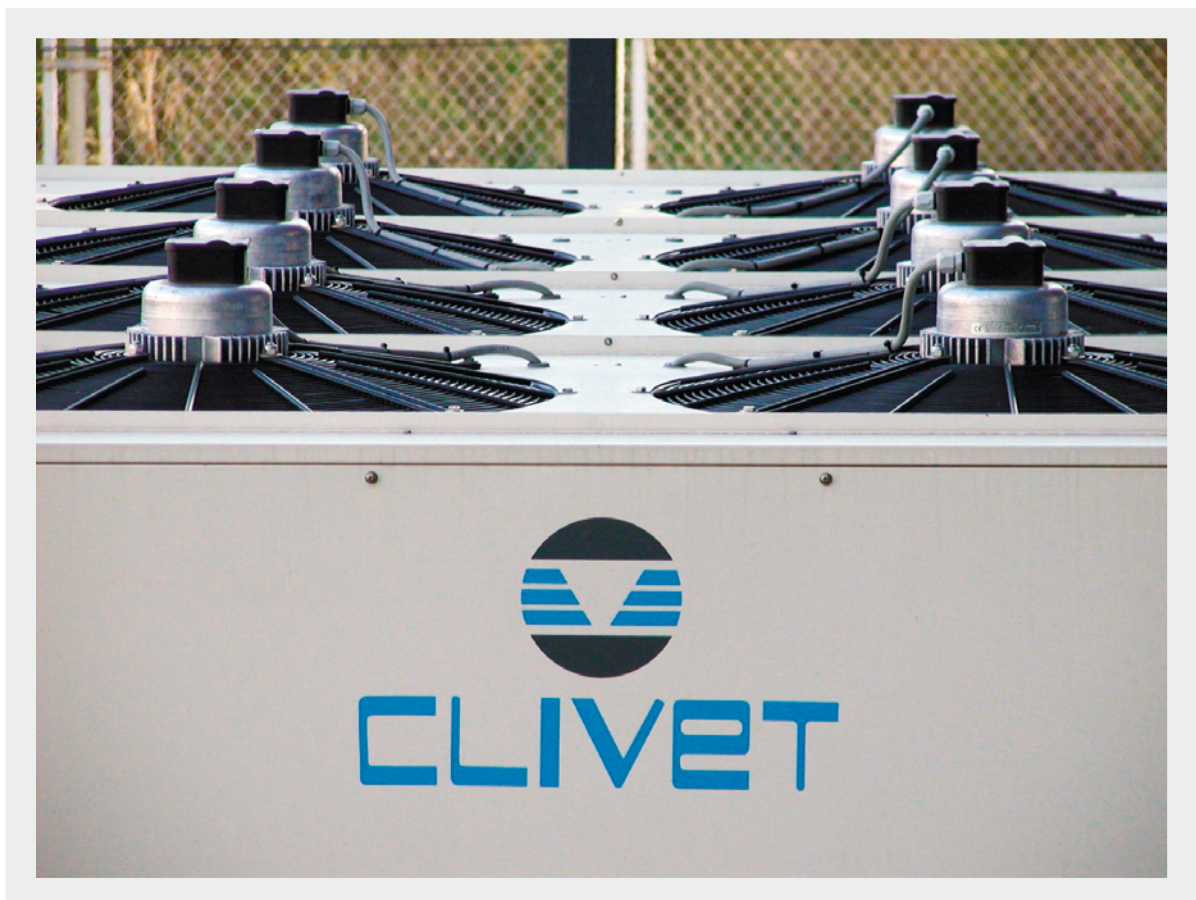
Air conditioning system
